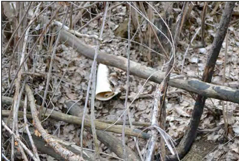
Photo B9: This pipe is located at the southwest corner of Area B. According to the property owner, Mr. J. F. Moore, this is an overflow wastewater pipe that allows him to pump wastewater from the canal into the ravine at his discretion.
