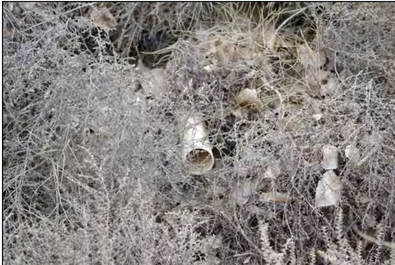
Photo B15: This photo is of the second pipe that supplies water to the pond.
