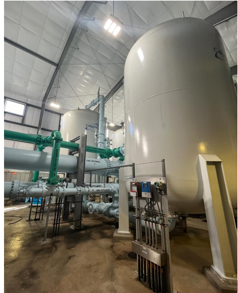
Example of GAC pressure vessels
