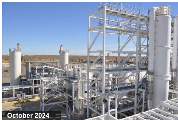
200 West Pump and Treat Facility
