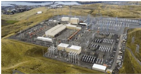
Pacific HVDC North Terminal near The Dalles
