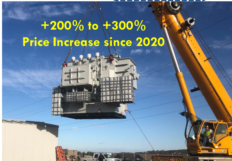
25-megawatt Substation Transformer
