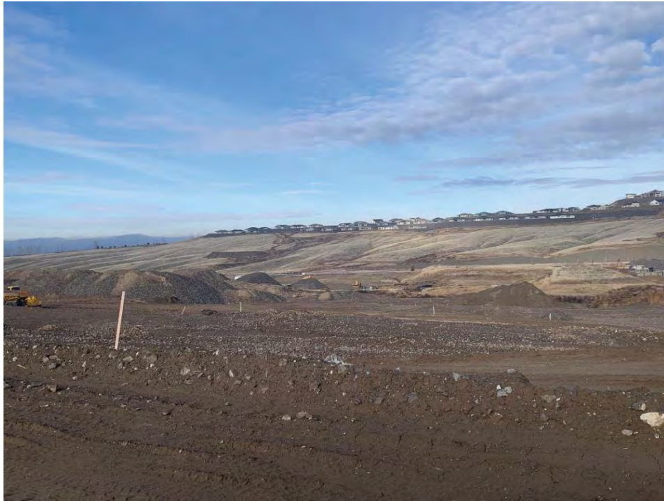
Figure 17. Overview of project area - note the white PVC pipe sticking out of the ground in the foreground (Aspect: Northwest).
